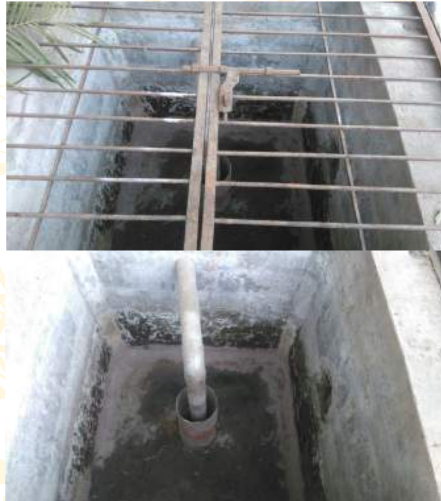
RAIN WATER HARVESTING SYSTEM
